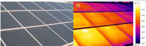
Not Every Hot Spot is a Defect – Thermograph of the Junction Boxes
